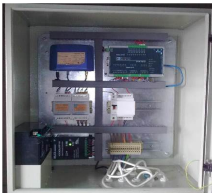
Slika 2. Realizovan autonomni sistem Figure 2. Implemented autonomous system
