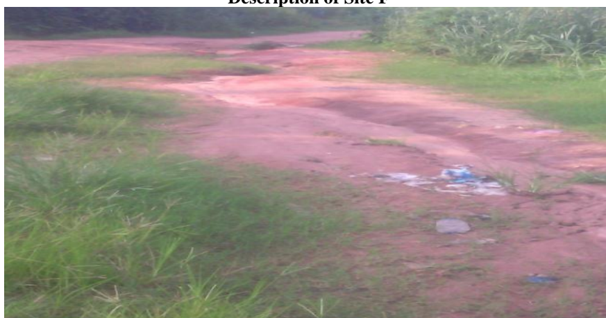
Plate 6: Erosion at site F
